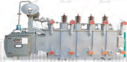
2500 kVA, 33/0.8 kV Inverter Transformer
